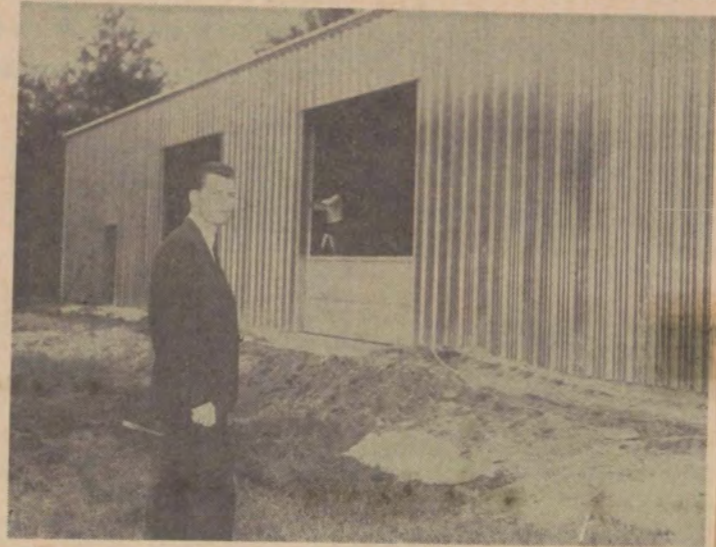
MACHINERY SHOP — Craig Allen of St. Pauls, director of the Robeson County Extension Unit of Fayetteville Technical Institute, stands in front of a new farm machinery shop under construction at the school, located in the Barker-Ten Mile community near Lumberton. (Observer photos—Wilson)
