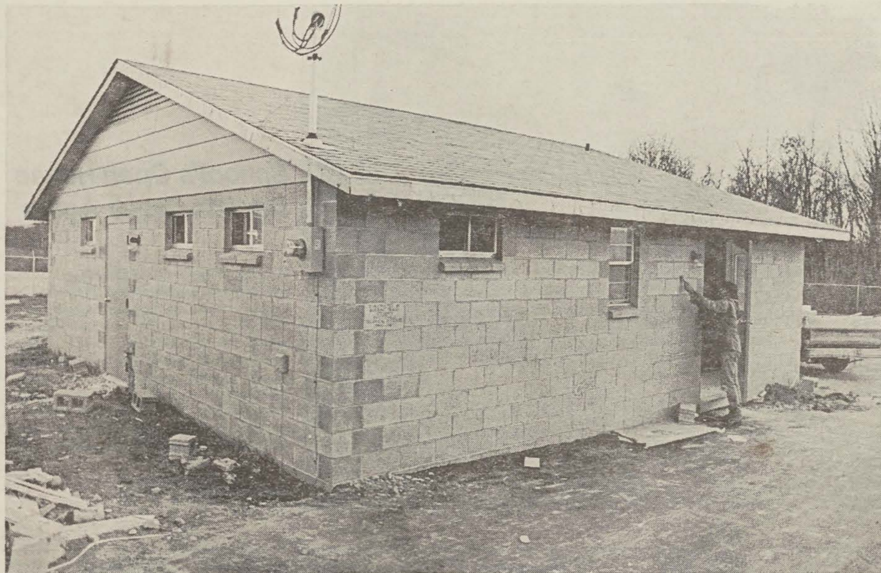
A Fayetteville Technical Institute student works on the Animal Haven shelter on Bragg Boulevard as it nears completion in this photo taken on Dec. 20, 1985. FTI students are expected to begin work on a new wing for the year-old shelter as funds become available.
