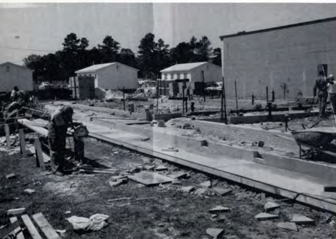
The plumbing and electrical Conduits are installed in foundations at rear addition to the building.
