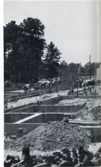
Forms removed from special tanks in foundations used for dynamic pump flow studies in Sanitary Engineering Lab.
