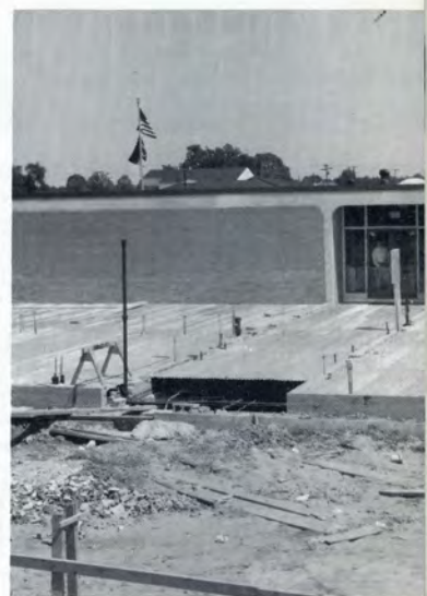
Forms, and Plumbing and Electrical conduits in place; Ready to pour the concrete floors on the West End Addition.
