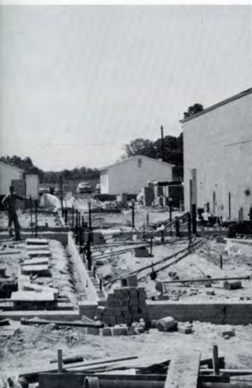
Special piping and conduits in place, ready to lay up walls and pour floors at rear addition to the building.
