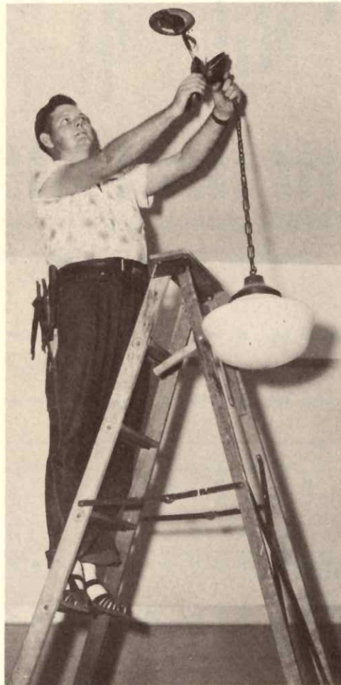
Planned relighting and rewiring incorporate better light with lower operating cost.
