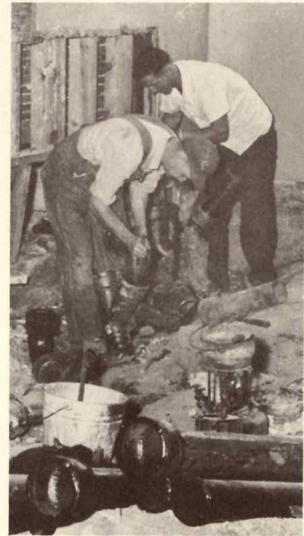
Toilet and remodeling schedules are providing facilities in keeping with health and cleanliness standards.
