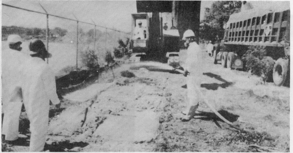
Officials of the Environmental Protection Agency clear Norwood site of toxic wastes called PCB's. This cleanup took place last spring.
