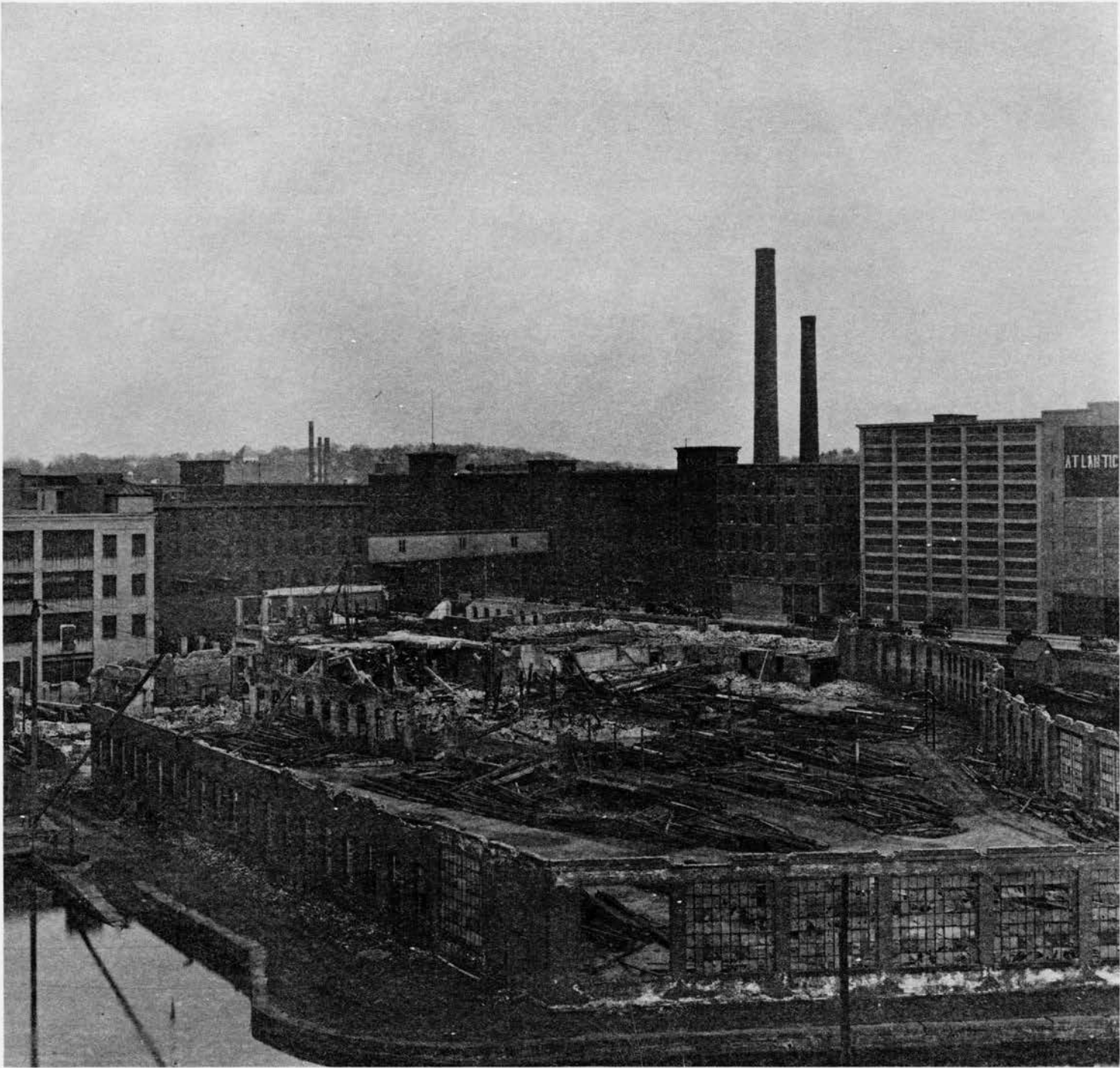
Figure 3-38 View of the foundry of the Lowell Machine Shop during demolition, ca. 1932.
