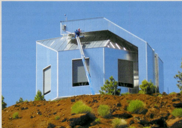
Construction workers have spent the summer putting the outside panels, shutters, seals, and finishing touches on the DCT dome.
