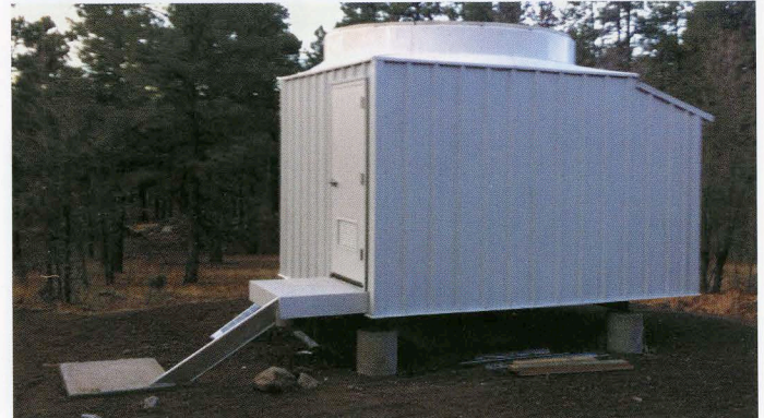
Fig. 3: The building is mostly complete and ready for installation of the fiberglass dome.
