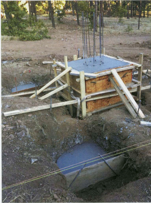
Fig. 1: The central pier to support the telescope includes a 4'x4'x4' cube of concrete sitting directly on bedrock. Each of the four building piers extends down to bedrock as well.
