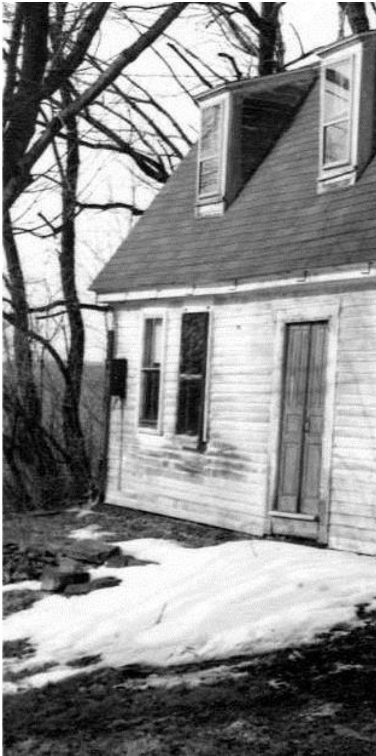
Figure C5a. Detail, Photograph ca. 1912 of Daniel Rose House showing the same double-leaf door and stonework later photographed in 2001 by Bill Phelon. Note elevation to west from west facing cellar wall containing what Bill Phelon believed to be gun portals for defense and signaling to Rose family members living east of brothers Daniel and David Rose. On the western slope of Prospect Mountain, the view west presented a defensive outlook. A stone foundation to support a palisade across the front of the house is evident here to the left of snow and still exists today. The Daniel Rose House is in the West Granville National Register Historic District. Perspective view, camera facing northwest.
