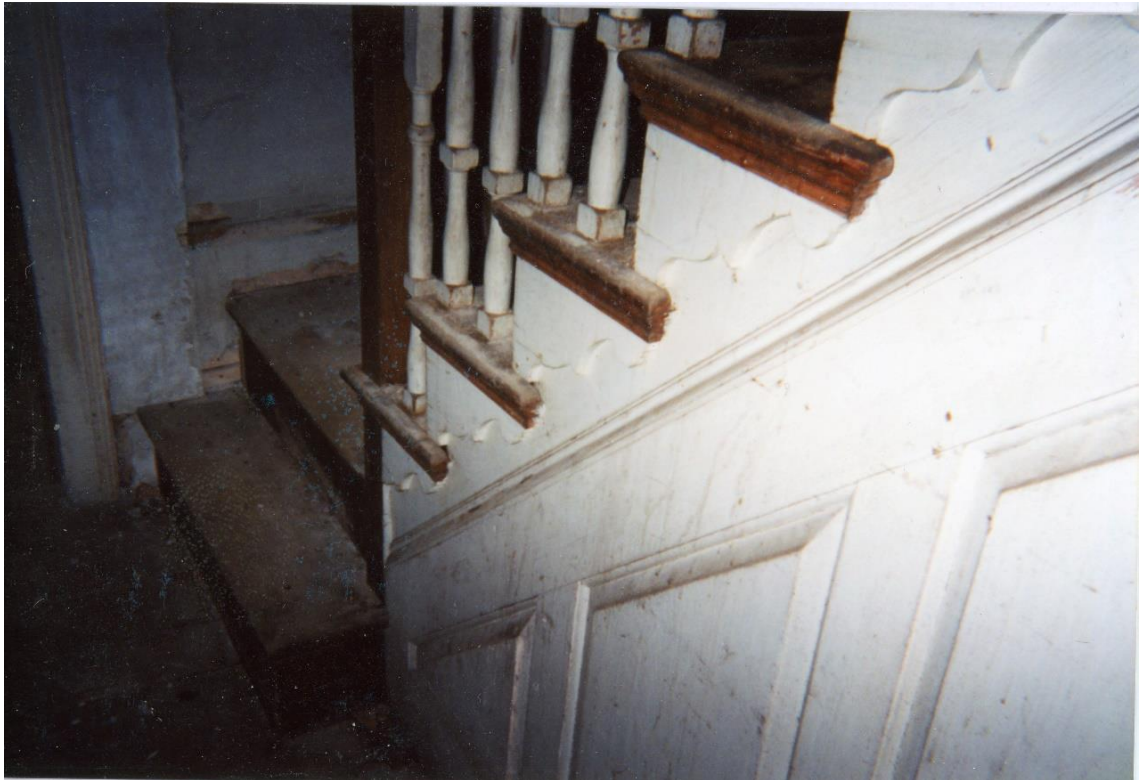
Figure 3.40. Pre-restoration, Daniel Rose House Front Hall “balustrade single landing staircase” as described in the 1985 Legacy Inventory, “with raised panels, turned rails and details along stair treads.” Paint analysis revealed green paint color on dado that was also originally used in the Front Southwest Parlor. (Upper) Camera facing east; (Lower) camera facing northwest with doorway to Front Southwest Parlor. Photos by William Brian “Bill” Phelon, ca. July 2004.
