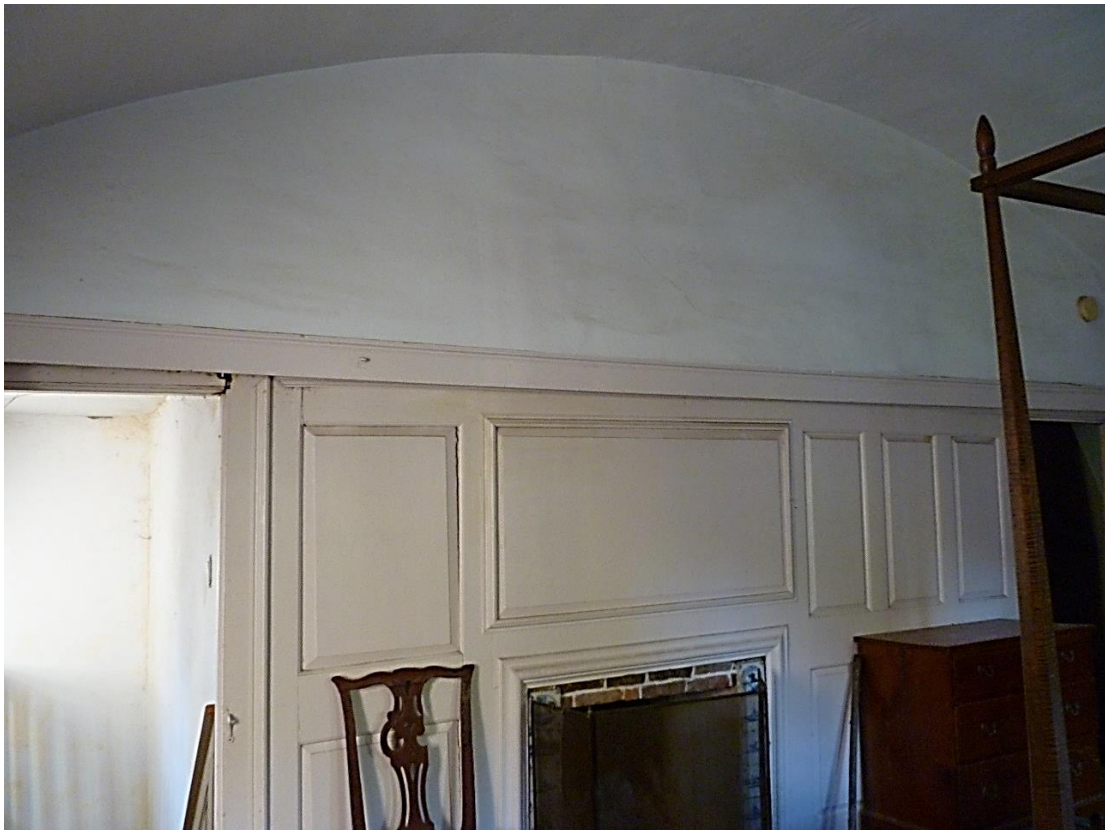
Figure 3.46. Ballroom, west breast wall, second-floor barrel vaulted ceiling rising to a height of twelve feet and evidencing blue paint pigment found in fallen ceiling plaster. Daniel Rose House 1741. Cameras facing northwest. Previously sealed doorway is to the left, to main stair landing and front entrance hall. (Upper) Photo, ca. July 2004. (Lower) Restoration by Bill Phelon. Photo, September 2019.
