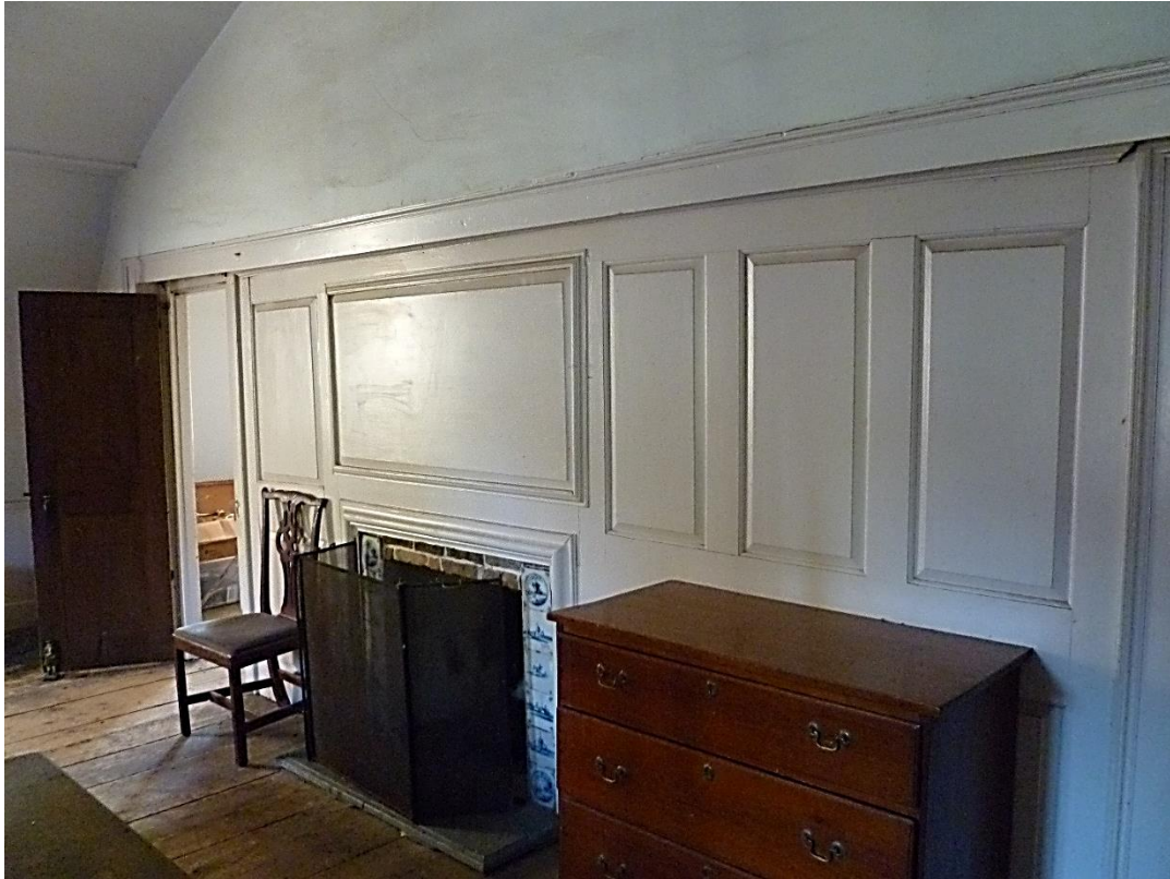
Figure 3.50. Ballroom, west breast wall. This Southeast Bed Chamber runs the entire width of the Daniel Rose House, with the barrel vaulted ceiling rising to a height of twelve feet. Restoration by Bill Phelon. Camera facing southwest, September 2019.
