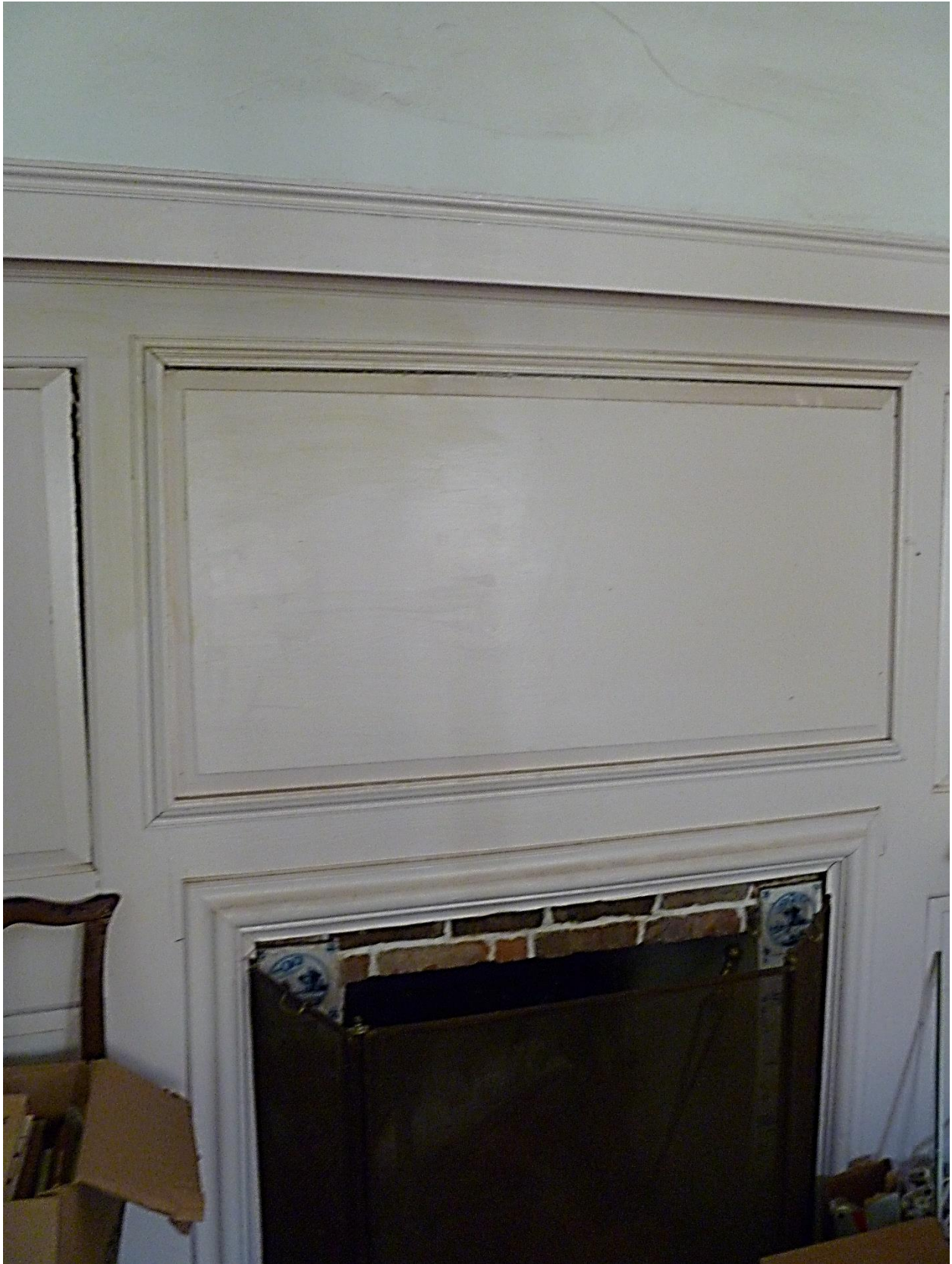
Figure 3.49. Front Southeast Bedchamber chimney breast wall with fielded panels and fireplace restored by Bill Phelon, Daniel Rose House, 1741. Camera facing west, September 2019.
