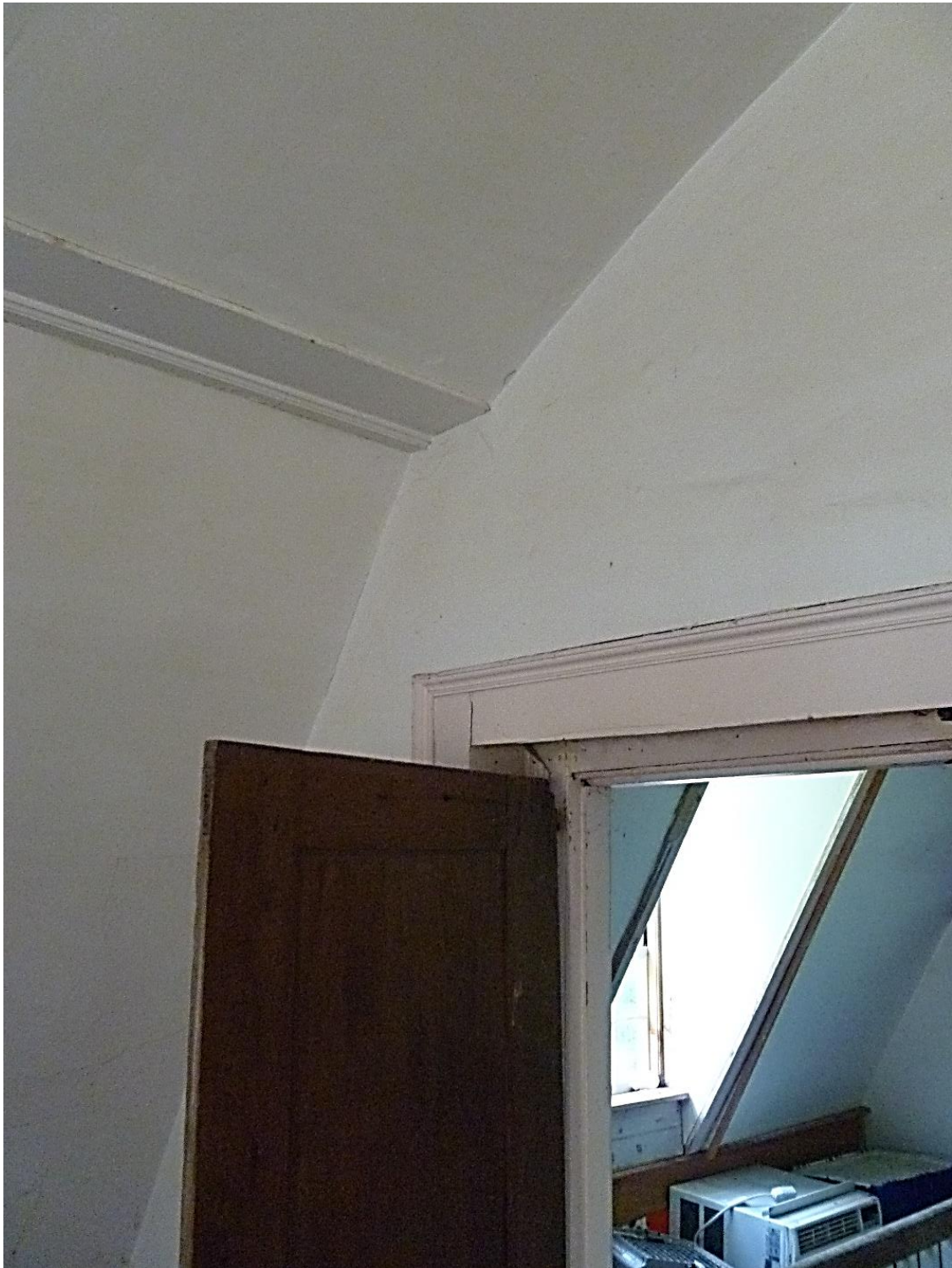
Figure 3.51. Front Southeast Bedchamber, Ballroom with barrel vaulted plaster ceiling, restored, ascending to twelve feet, Daniel Rose House. View to Stairway enclosure, center gable window and landing above front entryway. Camera facing southwest, September 2019.
