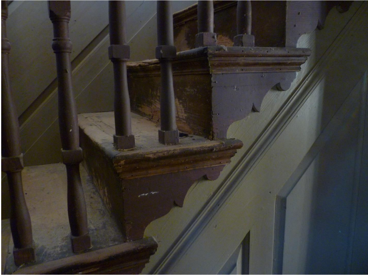
Figure 3.41. Daniel Rose House front hall “balustrade single landing staircase.” Layers of later paint removed from the rails, step details and dado; green paint color, also found in analysis of the Front Southwest Parlor, restored by Bill Phelon. Missing paneling and rail on fourth step, reconstructed and fitted to original locations. Camera facing north. Photo, September 2019.
