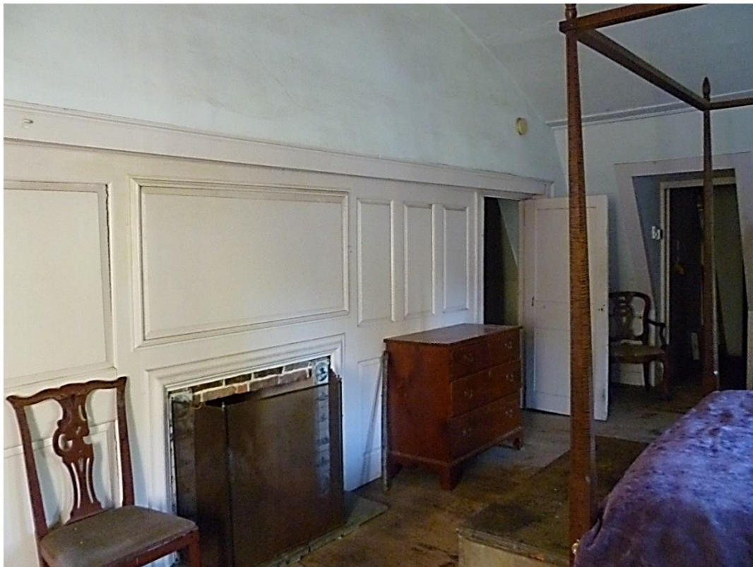
Figure 3.47. Ballroom, west breast wall and north gambrel wall with daylight evident during roof reconstruction and lathe in repair. Second-floor barrel vaulted ceiling rises to a height of twelve feet. Cameras facing northwest. (Upper) Photo, ca. July 2004. (Lower) Restoration by Bill Phelon. Photo, September 2019.
