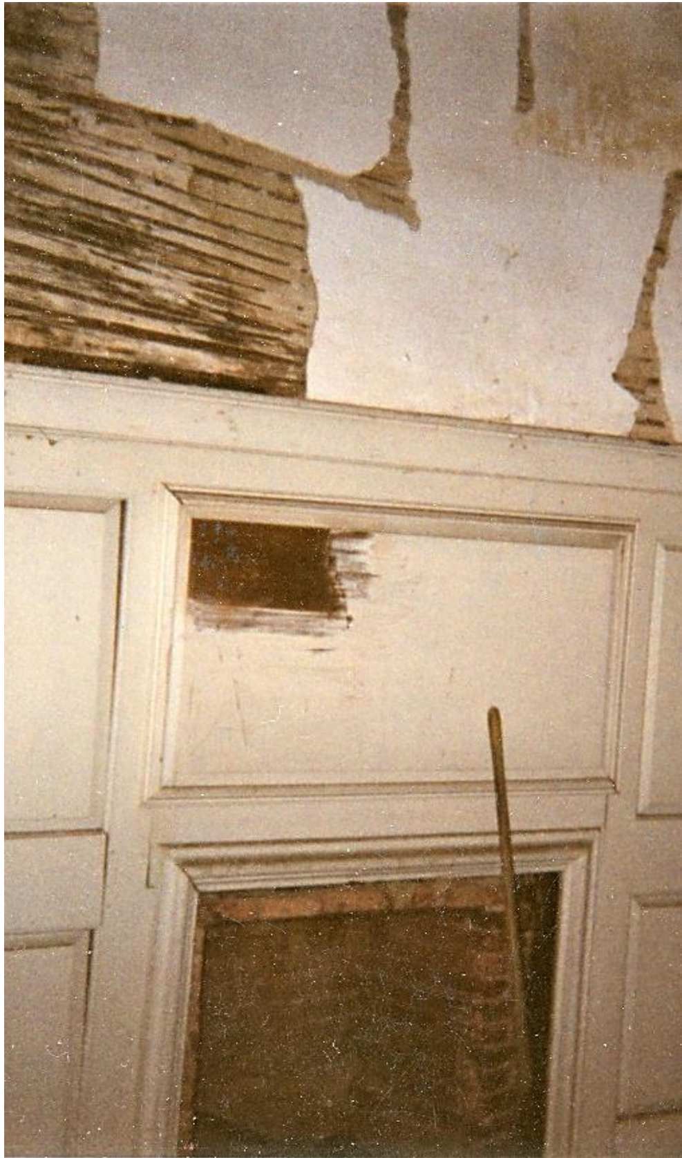
Figure 3.48. Front Southeast Bed Chamber, Ballroom, west breast wall of fielded panels. Fireplace brick evident. Pre-restoration; paint analysis. Camera facing west, ca. July 2004.
