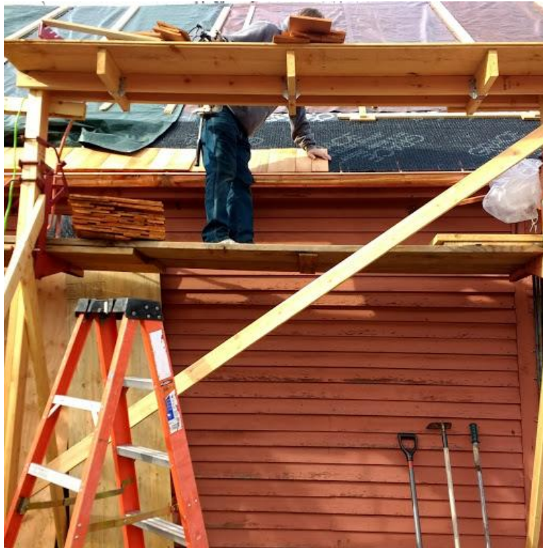
Figure 3.56a. In December 2017, a new roof was put on the two-story addition (ca. 1985) extending north from the keeping room, a potential ‘Docent Wing’: with Grace Ice and Water Shield underlayment, one layer of royal cedar breather and then two layers of red cedar perfection for “three sheets (of shingles) to the wind” in the old tradition with hand crafted gutters and leaders to last sixty plus years. Camera facing southwest. Photos, December 2017.
