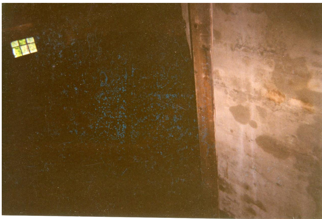
Figure 3.58. Attic (Upper) featuring mortise and pegged tenon construction (see peg, upper right) with (Lower) flat stone center chimney. Daniel Rose House, 1741. Camera facing six pane window, west elevation. Photos by Bill Phelon, ca. July 2004.
