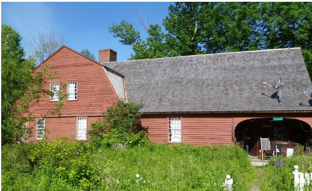
Figure 3.57. Daniel Rose House, 1741, east façade with new roof of three layers of cedar shingles added to the potential ‘Docent Wing’ in 2017. Photo, June 2019.
