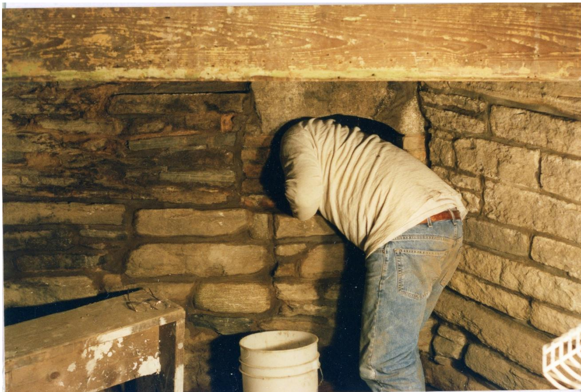
Figure 3.21. Keeping Room, Daniel Rose House, 1741. Bill Phelon at work completing the pointing of the brick interior of the bake oven. According to the Legacy Inventory of 1985, the fireplace is “built completely of flat stone.” According to Curtis, March 24, 2003: “The cavernous kitchen fireplace, with its stone firebox, bake oven situated at the rear, and provision for lug poles to be suspended within the flue, is a throwback to the early 18 th century.” Pre- (“12” and “13”) and post-restoration (Lower) photos, July 2004.
