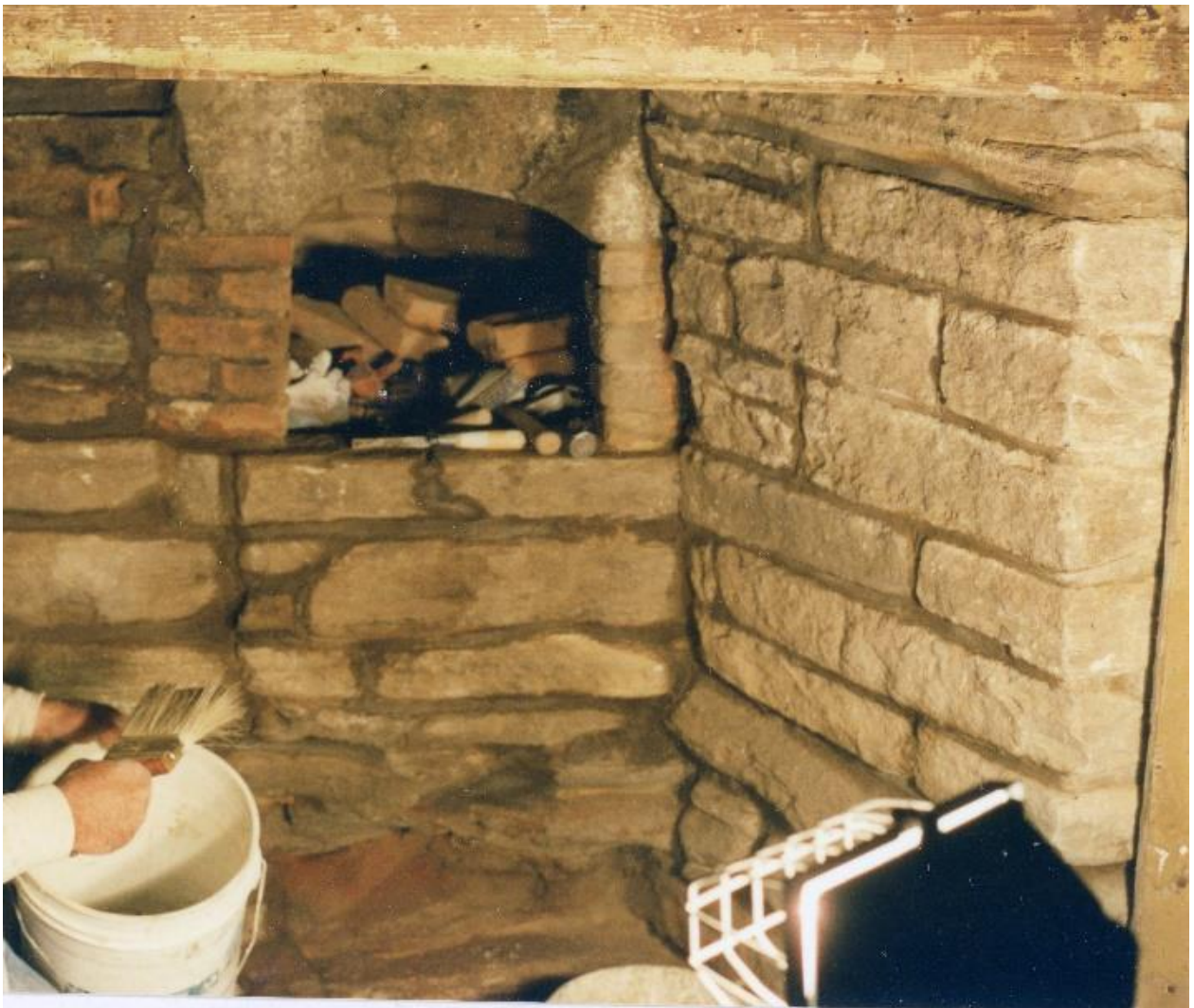
Figure 3.22. Keeping Room, Daniel Rose House, 1741. (Upper) Photo “14”: Pre-restoration assessment and preparation by a stone mason supervised by Bill Phelon; and (Lower) Restoration in progress. The stone lintel of the bake oven is supported by brick. The fireplace is built completely of flat stone with brick around and in the bake oven. Photos, July 2004.
