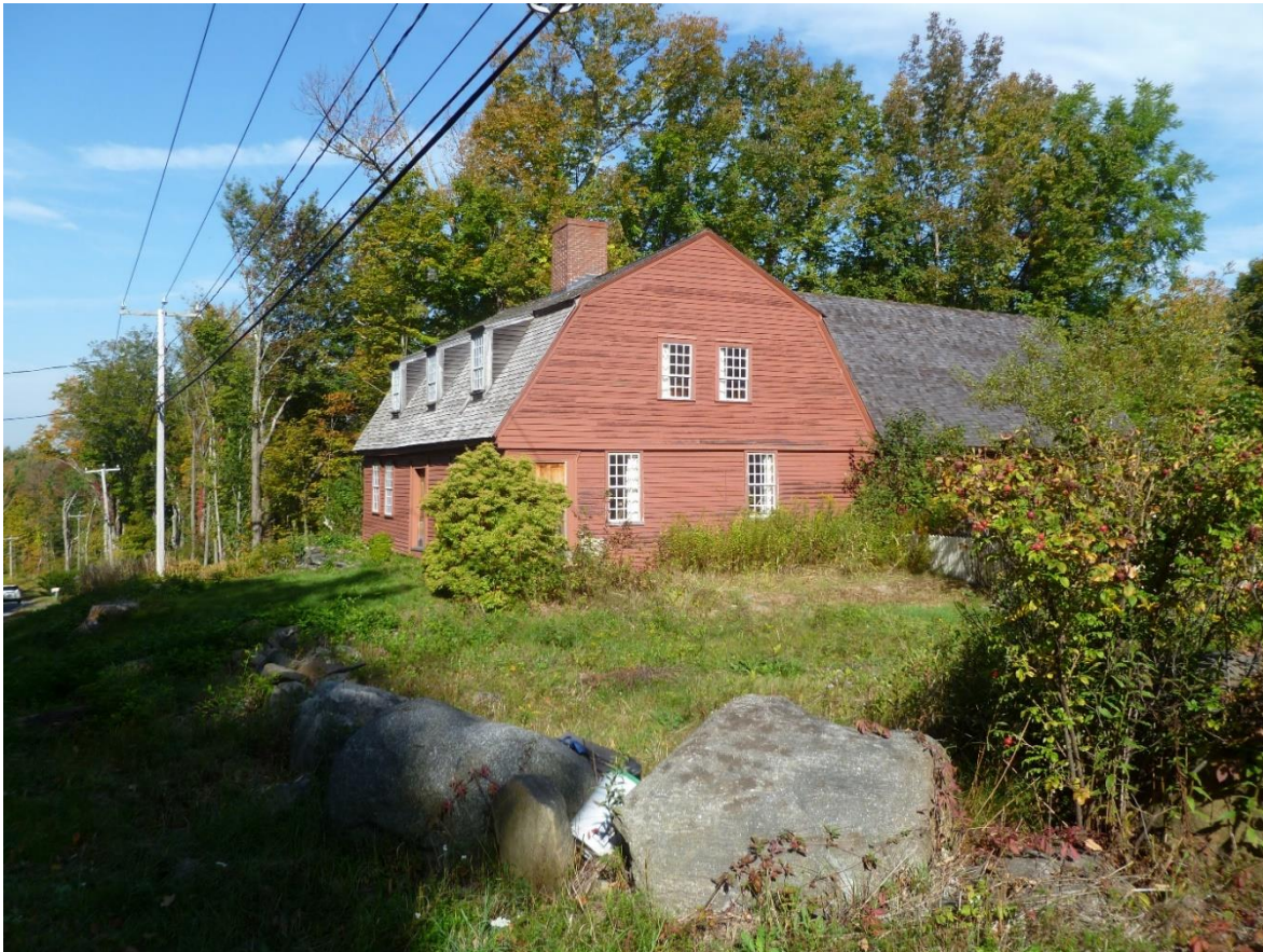
Figure 3.5. Daniel Rose House, 1741. Camera facing northwest, June 2001. (Lower) Bill Phelon restored the cedar shingle roof on main house and twentieth-century potential ‘Docent Wing’ (living quarters for a Museum caretaker’s family) to the north. Photo, September 2019. The Rose-Baldwin-Baker-Phelon House is in the West Granville National Register Historic District (sign just east of house near eastern line of Daniel Rose’s original settlement lot intact in 1985).
