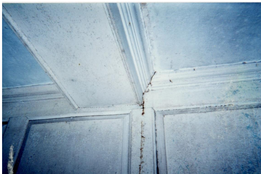
Figure 3.39. Pre-restoration Southwest Front Parlor, Daniel Rose House. According to the Legacy Inventory, 1985, the “Perimeter is covered with wood panel dado plaster above. Ceiling beams, summer beams and corner post are cased and molded. Floors are wide pine boards original.” This was originally the room allocated for Denizen Baldwin in the court settlement of his father Lt. Jacob Baldwin’s estate in 1813. Denizen served as a U.S. Navy Master’s Mate in the War of 1812 aboard the victorious USS Peacock , which defeated HMS Epervier and by his action merited a Congressional presentation sword in 1814, considered one of the finest known. (Upper) Camera facing southwest, 2004. (Lower) Summer beam above fireplace breast wall: notice same crack and cream color paint (photo development blue color is inaccurate) in previous photos. Color analysis indicated original green paint on woodwork, as also found in the front hallway. Camera facing east, 2004.
