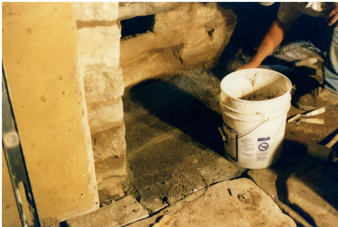
Figure 3.25. Keeping Room Hearth stone restoration, Daniel Rose House, 1741. Restoration by Bill Phelon, pointing the flat stonework after reinforcing and replacing, as needed, the supporting structure. The fireplace is extremely large and can fit two or three people in it at one time. Camera facing south (bake oven to right). Photo, July 2004.
