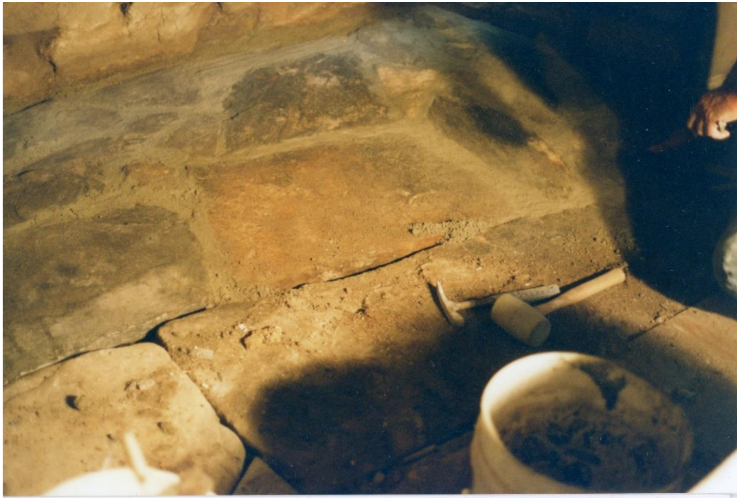
Figure 3.26. Keeping Room Hearth stone restoration by Bill Phelon at the Daniel Rose House, 1741. The fireplace is extremely large and can fit two or three people in it at one time. Photos, July 2004. Camera facing east (upper left) and west (upper right).
