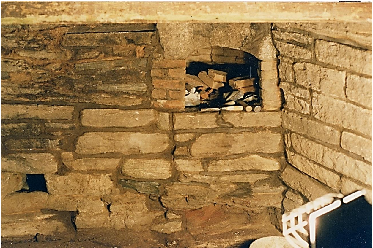
Figure 3.20. Keeping Room, Daniel Rose House, 1741. (Upper) Pre- and (Lower) restoration of the hearth and bake oven in progress (with mason's trowel, upper right photo; and chisels). Wood lintel of fireplace is across the top of photo; the bake oven has a stone lintel supported by brick. Photo, July 2004.
