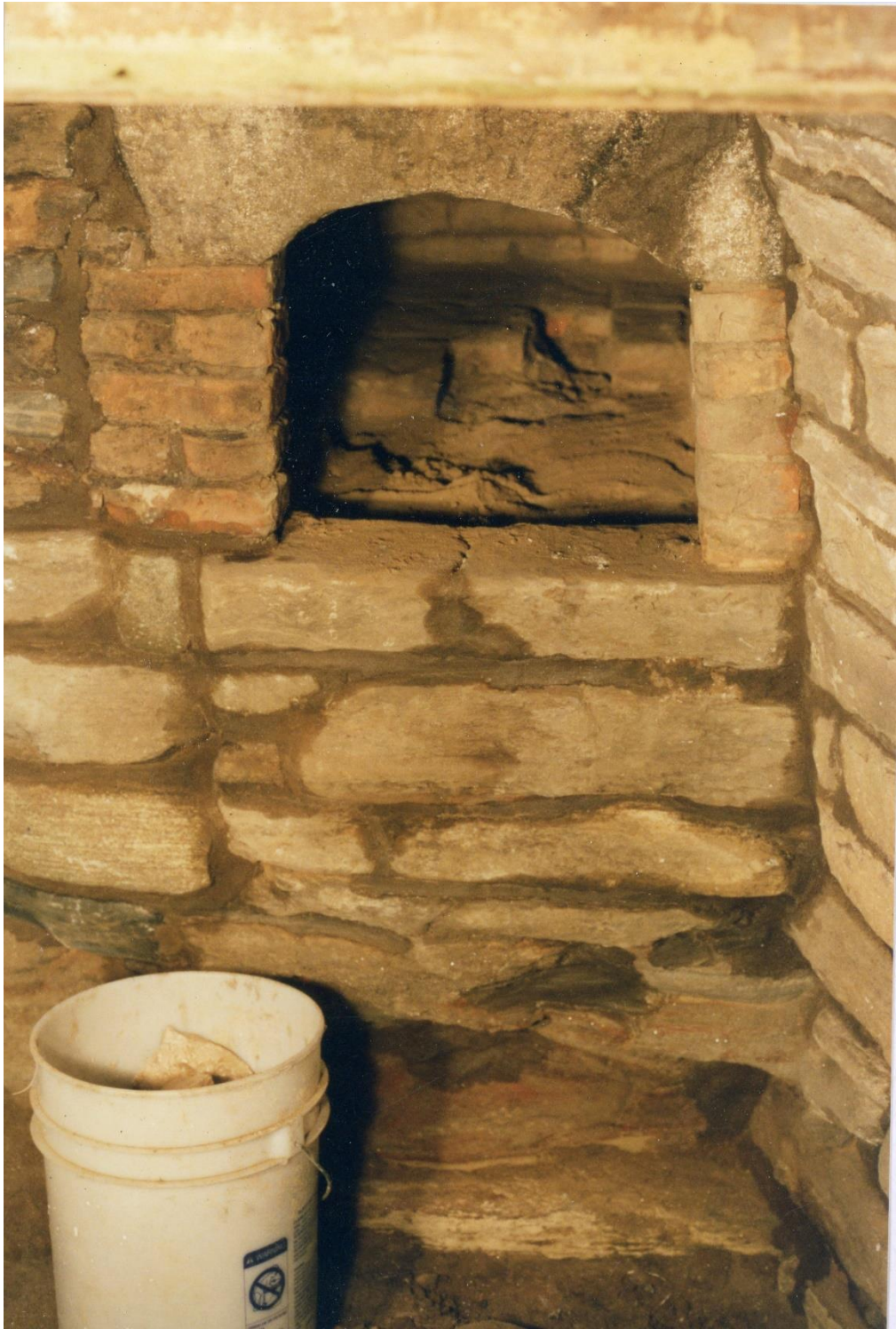
Figure 3.23. Keeping Room, Daniel Rose House, 1741. Restoration in progress. The stone lintel of the bake oven is supported by brick. The bake oven is lined with brick as restored by Bill Phelon. The fireplace is built completely of flat stone. Photo, July 2004.
