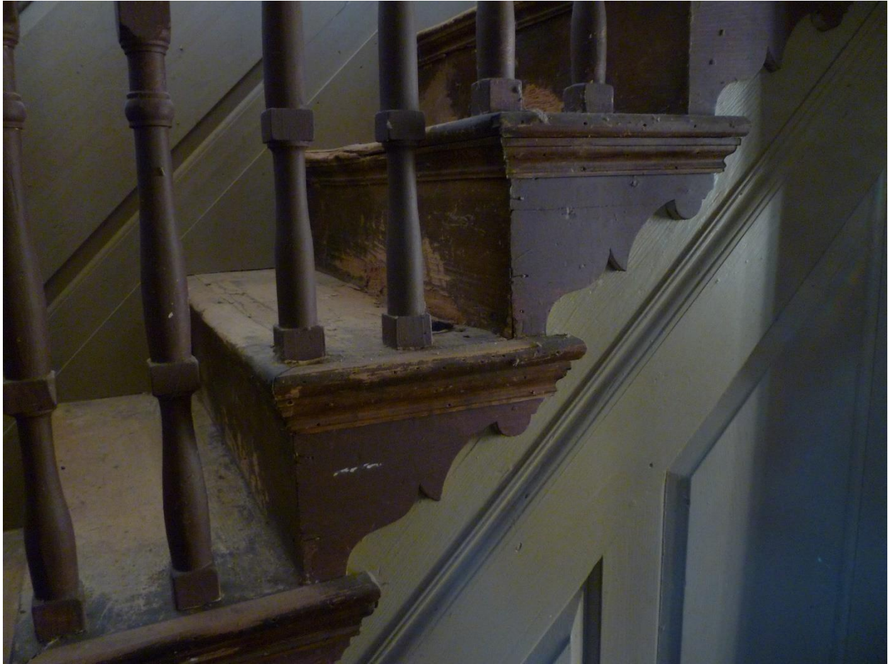
Figure 62. Front Hall with restored raised panels, turned rails and details on stair treads, parallel to front façade. Daniel Rose House. Camera facing north. September 2019.
