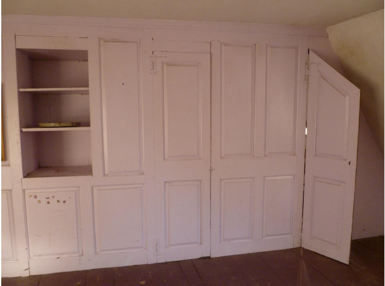
Figures 70. Bedchamber, second floor breastwall with closet revealing flat stone structure of center chimney, Daniel Rose House. Note "original white pine wide board floor" according to the MACRIS database inventory. Camera facing east. June 2019.
