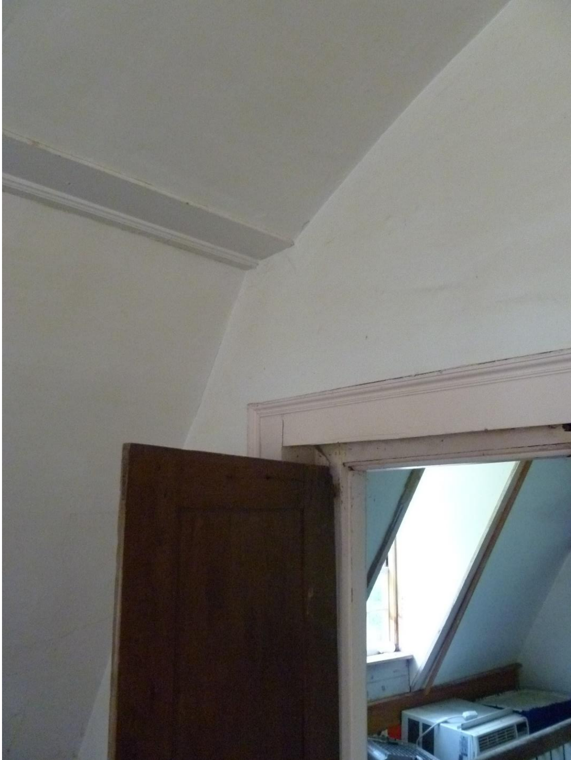
Figure 65. Front Southeast Bedchamber Ballroom with barrel vaulted plaster ceiling, restored, ascending to twelve feet, Daniel Rose House. View to Stairway enclosure, center gable window and landing above front entryway. Camera facing southwest.
