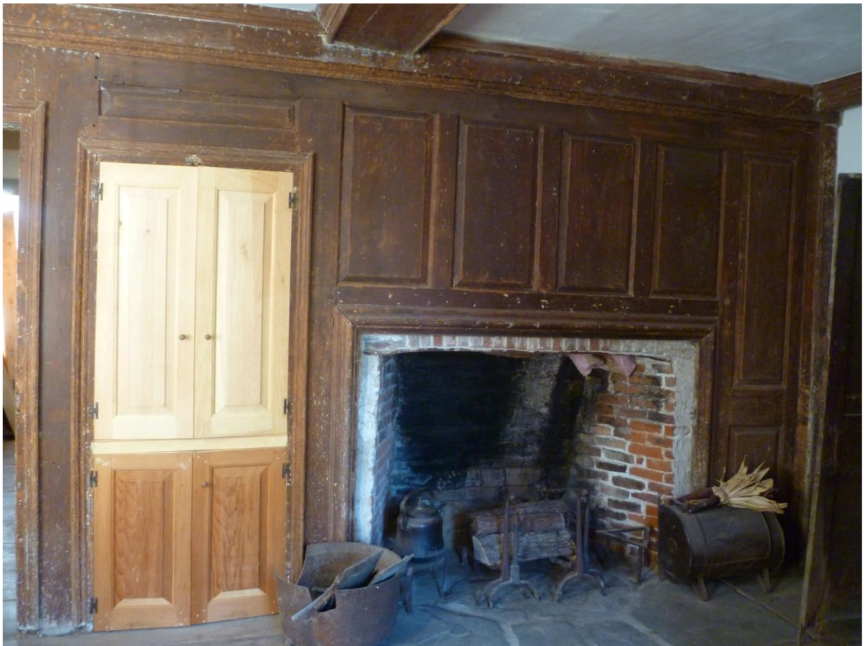
Figure 46. Southeast Front Parlor and Tavern Room, Chimney breastwall with raised panels were restored by Bill Phelon and cupboard doors were reconstructed, with old hinge marks still extant for proportion. Front hall is through door to the left. Camera facing west.
