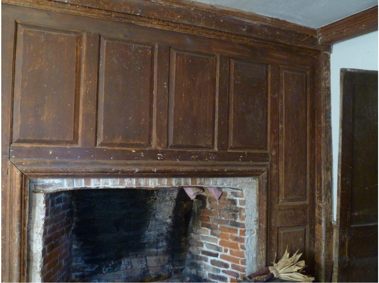
Figure 44. Southeast Front Parlor chimney breastwall with raised panels, restored by Bill Phelon, Daniel Rose House. Camera facing northwest. September 2019.
