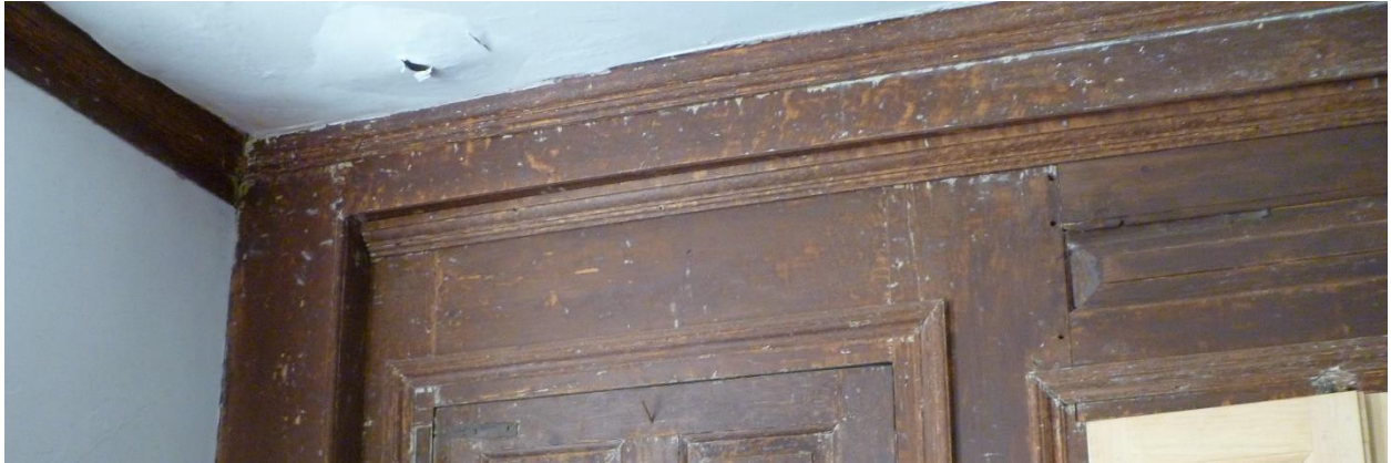
Figure 45. Detail, corner posts. Southeast Front Parlor chimney breastwall with raised panels above door to center hall, restored by Bill Phelon. Daniel Rose House. Camera facing southwest. September 2019.
