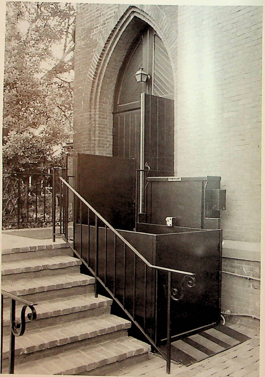
The Seminary chapel has become more accessible with the installation of an electric wheelchair lift at the front door.
