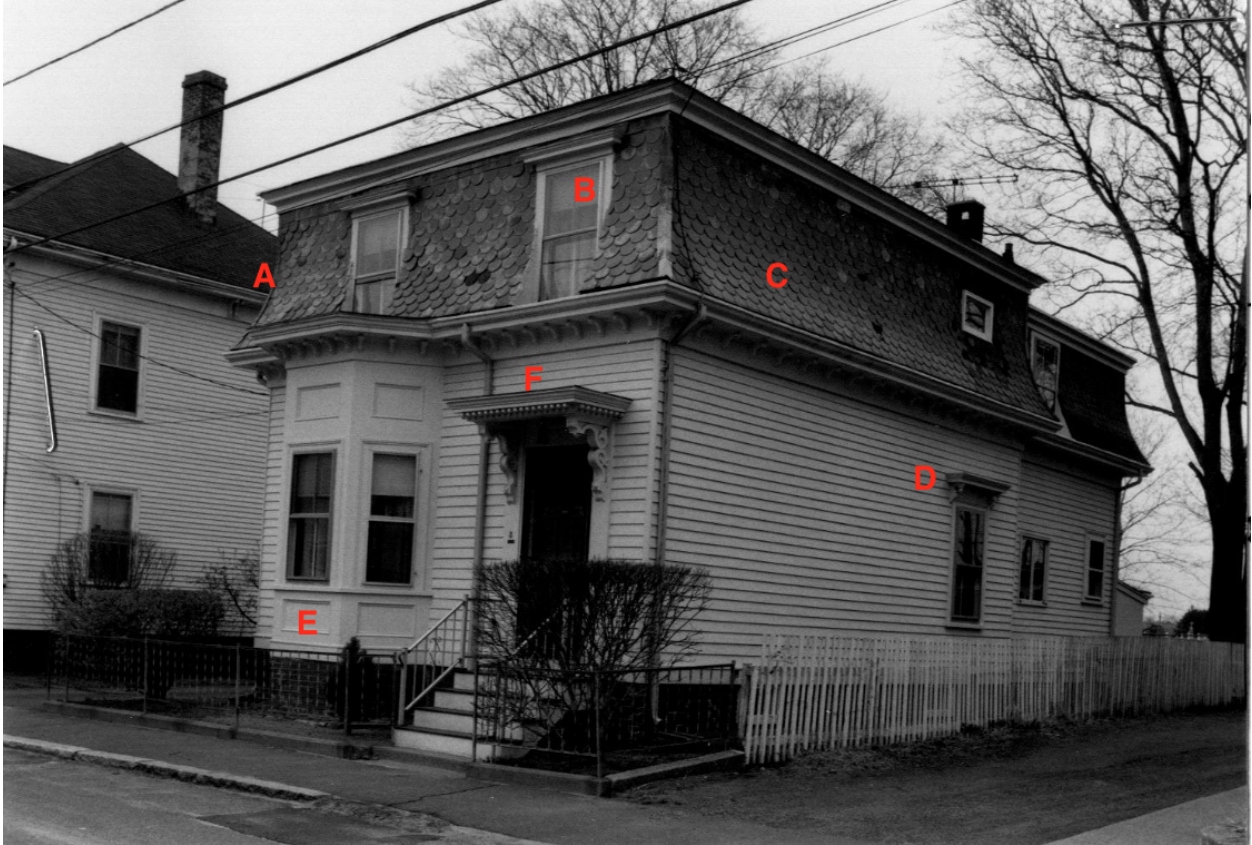
A 1986 picture of the house at 3 Woodside St. taken by Debra Hilbert of the Northfields Preservation Association. Much of the following analysis is borrowed from her notes. 62
