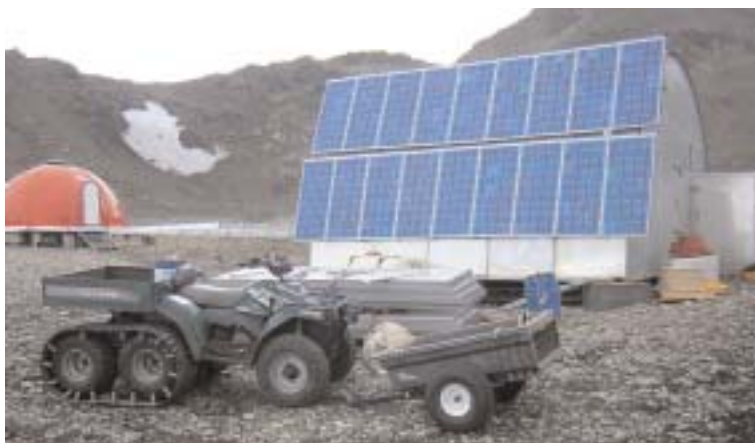
Photovoltaic panel banks at Juan Carlos I.
