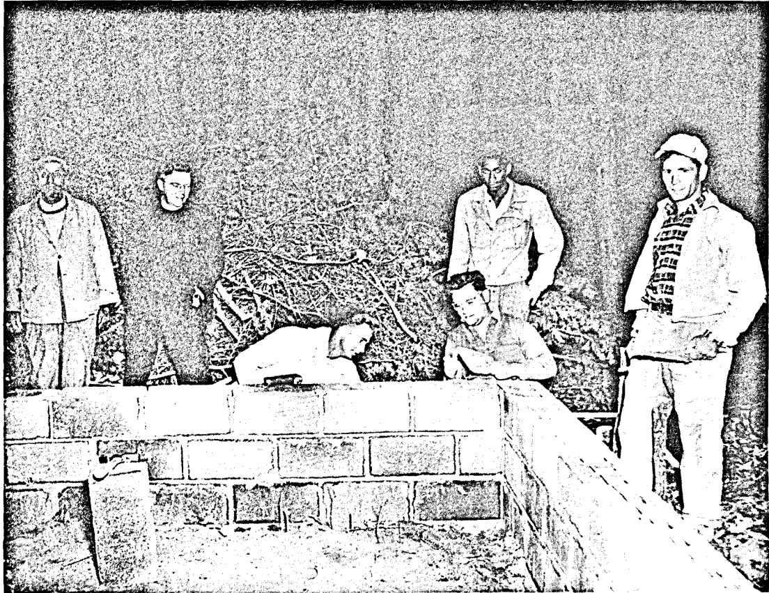
Bricklayers from Baltimore pitch in after work hours and build the walls for the home of Mr. John Ernest Berry. Here Father Kavanagh, Mr. Scanlon Herbert and Mr. Berry watch the work.
