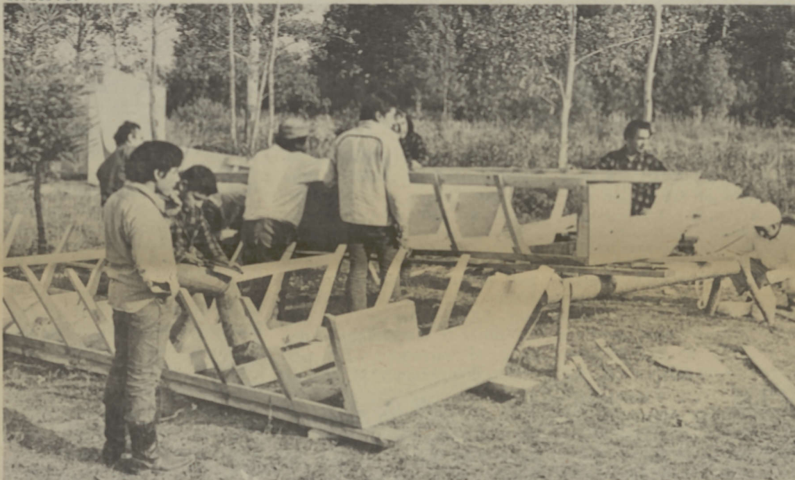
The twenty boats, which are being constructed at the site of the proposed resort, vary in lengths of 16 to 18 feet. Five of the boats will be used at the resort while the remaining fifteen will be shipped to northern Reserves in Saskatchewan to be used in commercial fishing. The boats at the resort will be used for tourist fishing in summer and for commercial fishing in the spring and fall seasons. The Band hopes a Commercial Fishing Co-operative will commence this fall on the Reserve.
