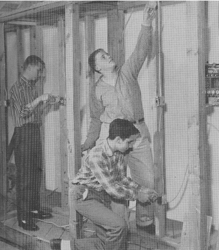
Wiring "mock" rooms are future electricians Gary Graeff, Leslie Saylor, and Charles Richter. They are cautious not to overload the circuit because they might blow a fuse.
