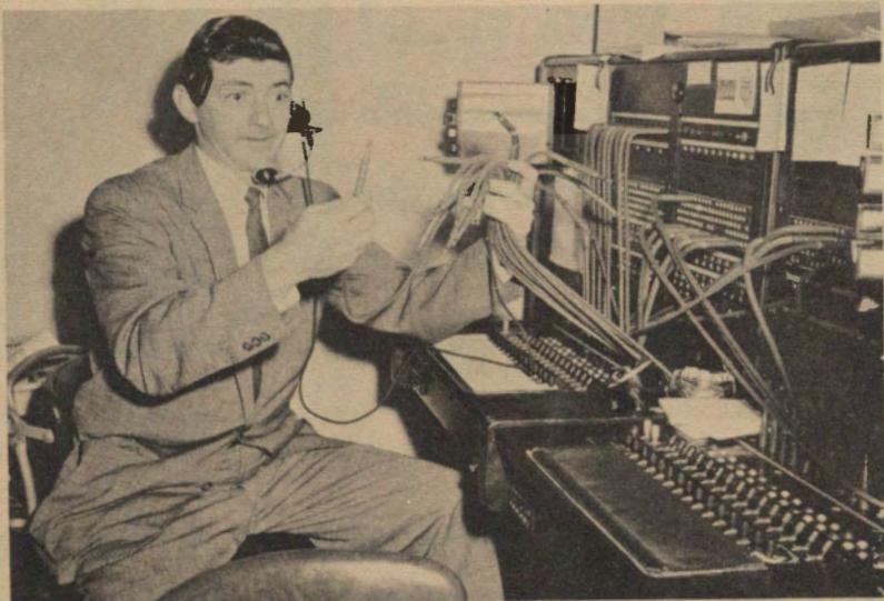
Assistant underwriting manager Lew Burritt, Jr., of the Chicago regional office took over switchboard duties while the ladies had their day and found himself temporarily confused by the maze of wires and cables.
