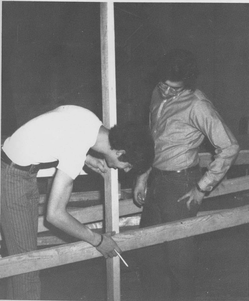
Mike Cooper and Rick Klein determine the best angle of construction to give the prop greatest stability.
