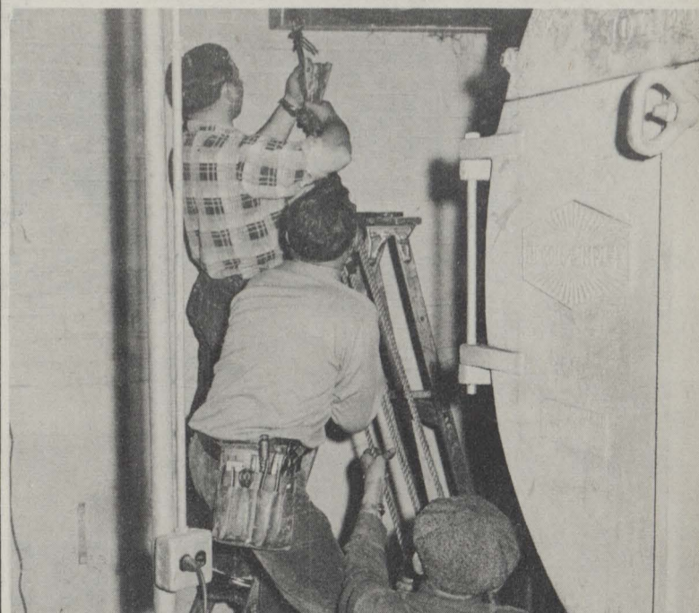
Workmen recently revamped the fire protection system at Cleveland School in Skokie.
