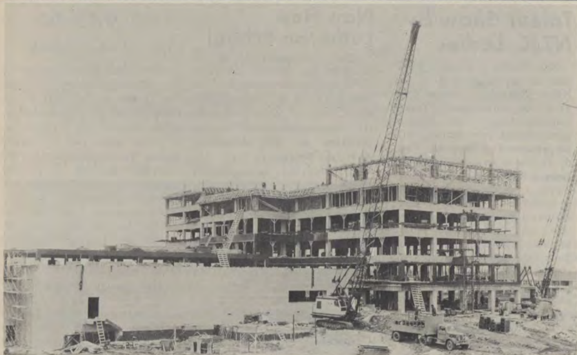
Construction work on Lutheran General Hospital and its school of nursing is ahead of schedule. Under construction on a 34-acre site at Western Avenue and Dempster Street in Park Ridge since April, the 326 bed general hospital and its school of nursing will be serving the residents and industries of the northwest area by the end of 1959. The cost of the project is $6,250,000 of which $1,375,000 was a grant from the federal government.
