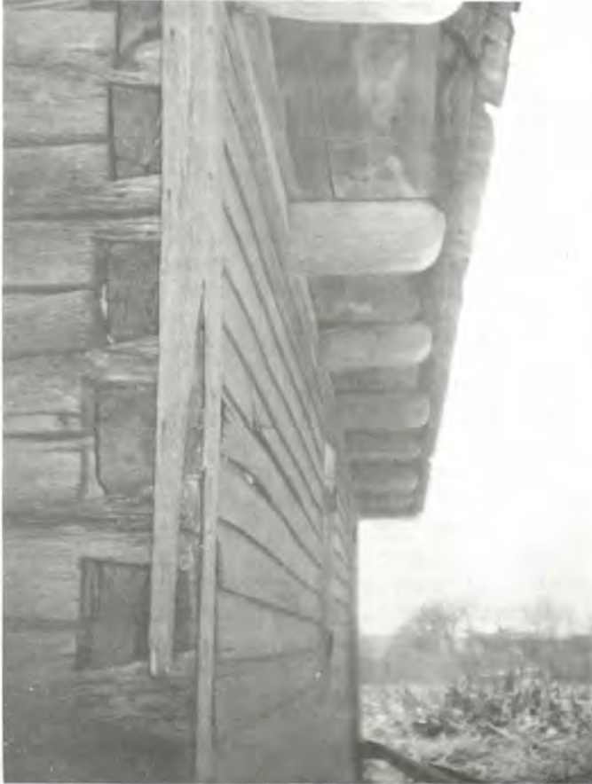
Lap siding attached long after original construction added years to the life of the structure's hand hewed log walls by affording protection from wind and rain.
