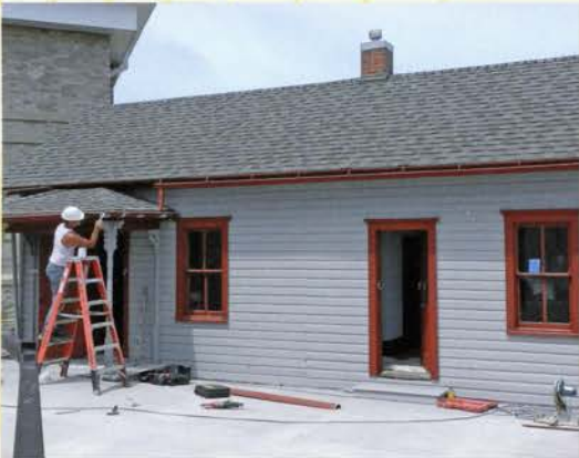
A worker from Roger Gwinnup Construction paints the exterior of the Sleger Immigrant Home its original color. Layers of paint were stripped from the house, both outside and inside, to find the true 1800s colors.
