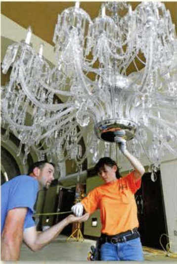
Judi Lynch, from Paulson Electric (right), secures a wire cover to the chandelier. There are 48 environmentally-friendly light bulbs in the chandelier. Three-watt LED bulbs will draw a total of 144 watts compared to the previous 1,920 watts of electricity. Nine people worked on the chandelier over four days. Fully assembled, the chandelier weighs about 500 pounds and is eight feet tall.
