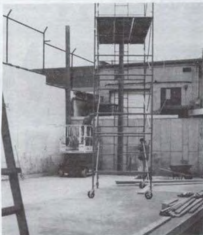
Photos: Mark Arellano and Mike Hinrichsen of Hinrichsen Construction at work on expansion of Omaha Mining Company
