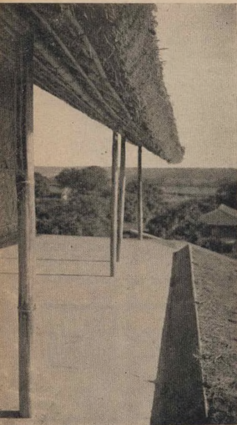
3. THE BUNGALOW VERANDAH, showing structural arrangement of bamboo posts and lintels, the woven bamboo wall panels and the encircling gutter. The eaves are brought well down to protect the wall from driving rains.
