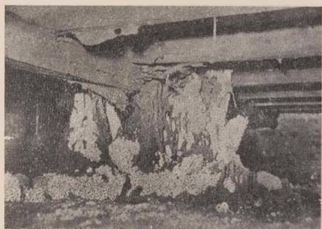
Fig. 11. Nest of Termes Badius in open unventilated air space below a suspended floor.
