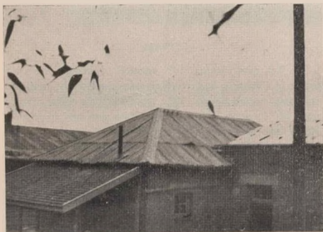
2. Contrast between corrugated asbestos, corrugated iron and South African pine shingles. Note the holes in the asbestos in several places. The corrugated iron is badly dented and loosened whereas shingles on the left were not damaged.
