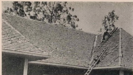
7. Portion of the roof of the wood Museum Building showing hail damage to shingles made of poor grade timber.
