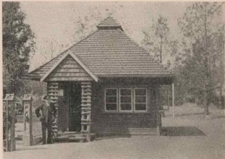
6. The same lodge, September 1950. Except for a few broken shingles, due to a severe hailstorm in November 1949, the roof is still in excellent condition.
