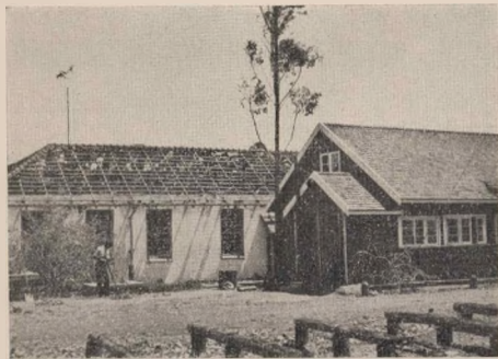
1. AFTER THE HAILSTORM IN PRETORIA, NOVEMBER 1949. Roof in the background was of tiles and that in the foreground is of South African pine shingles. The tile roof was completely smashed whereas the shingle roof suffered hardly any damage.
