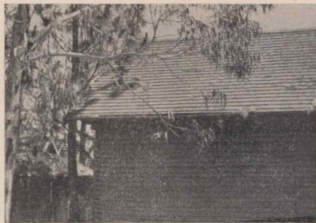
4. South face of cypress roof of log cabin which took the brunt of the November 1949 hailstorm. The roof suffered no damage and is in excellent condition although it had had seventeen years' service.
