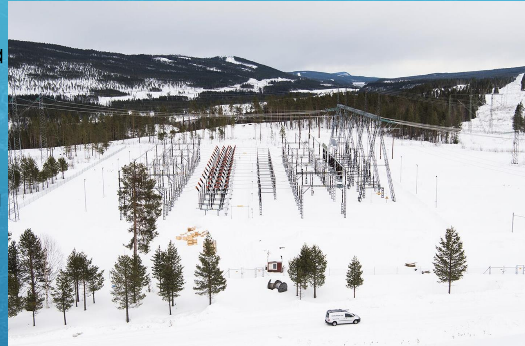
Power station outside Jokkmokk (Photo reportage: Coping with energy poverty across Europe | by The Beam | TheBeamMagazine | Medium )
