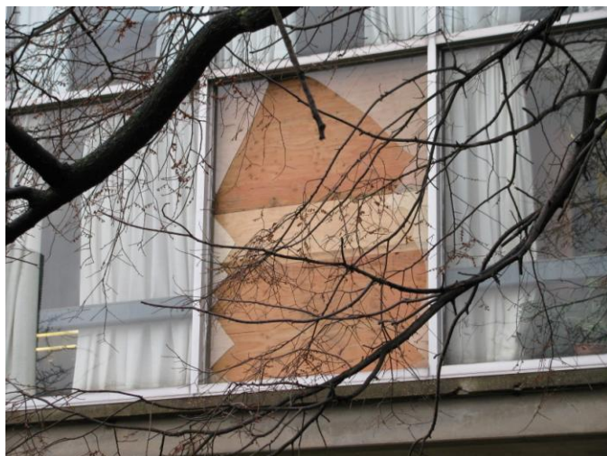
Broken window in the Library.
