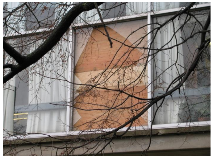
Broken window in the Library.
