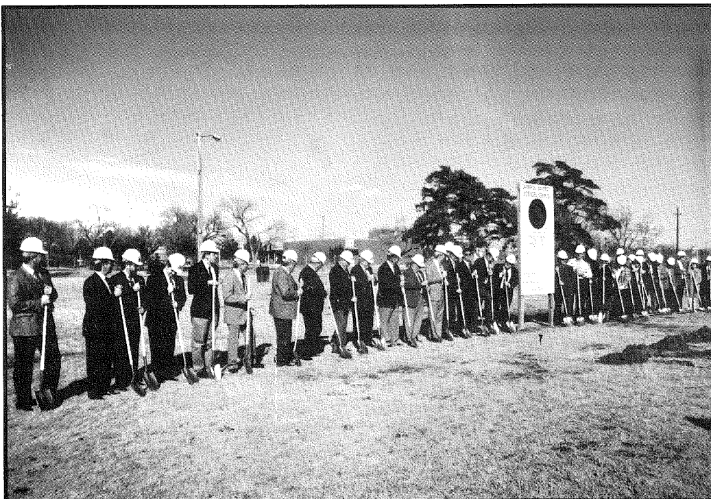
Dignitaries line up to break ground for Cameron University's new Sciences Complex. The two story 99,000 square feet facility will have a 110 seat auditorium, eight classrooms, 21 offices for faculty and state-of-the-art labs for physics, chemistry and biology.
