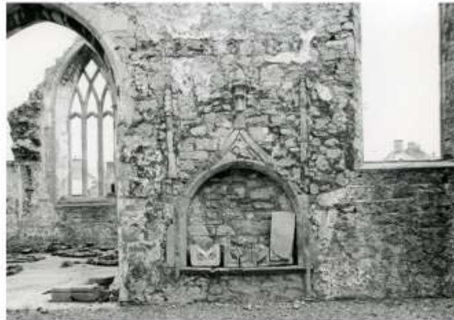
Ennis Franciscan Friary, tomb niche in the south nave wall. The mouldings and overall design of this niche suggest architectural connections with other sites in Clare, along with sites in Limerick, Kerry and Galway.
