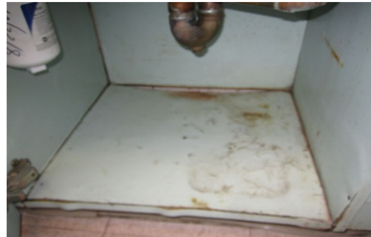
Leaks under sink and mold build up inside cabinet
