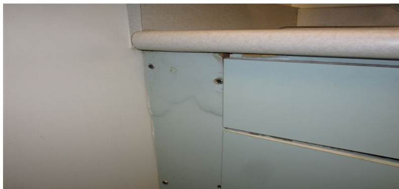
Example of Bolted Cabinets underneath sinks in patient care areas
