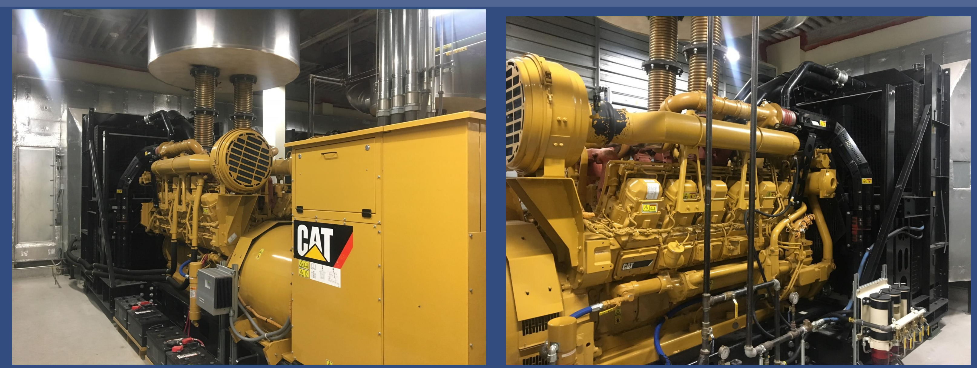
East Campus Generators
