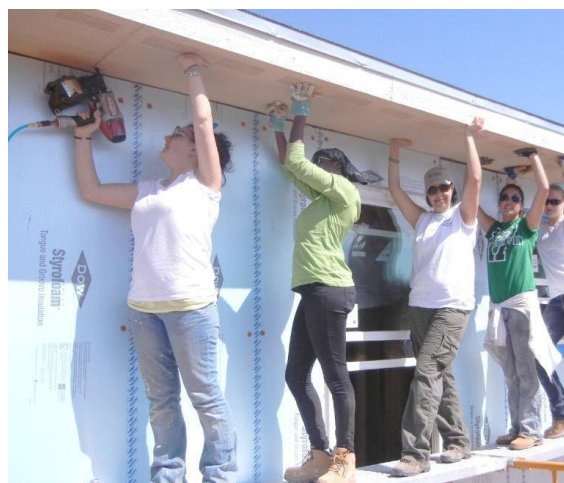
Kathleen Peets, third from left, works alongside students building a Habitat for Humanity home in Texas.
