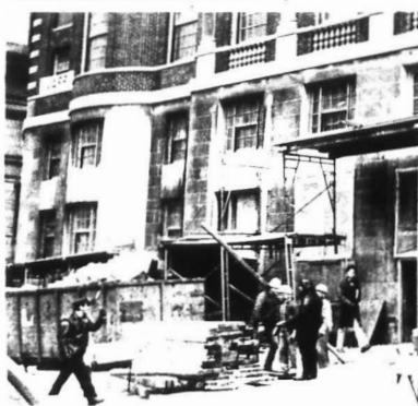
THE CONSTRUCTION GOES ON as it is now predicted that the Ashburton Place building will open in July
