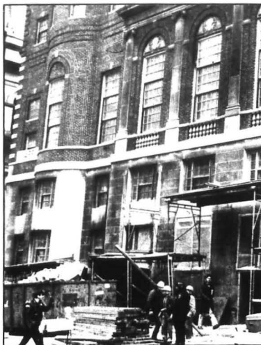
Construction work (above left) being done on Ashburton Place Building last year. Side entrance of the building (above right) that was specially built for President Calvin Coolidge so he could leave and enter the building, then the Boston City Club, undetected. Artists rendition (below right) of the lobby of Ashburton Place which should be completed soon, according to reports.
